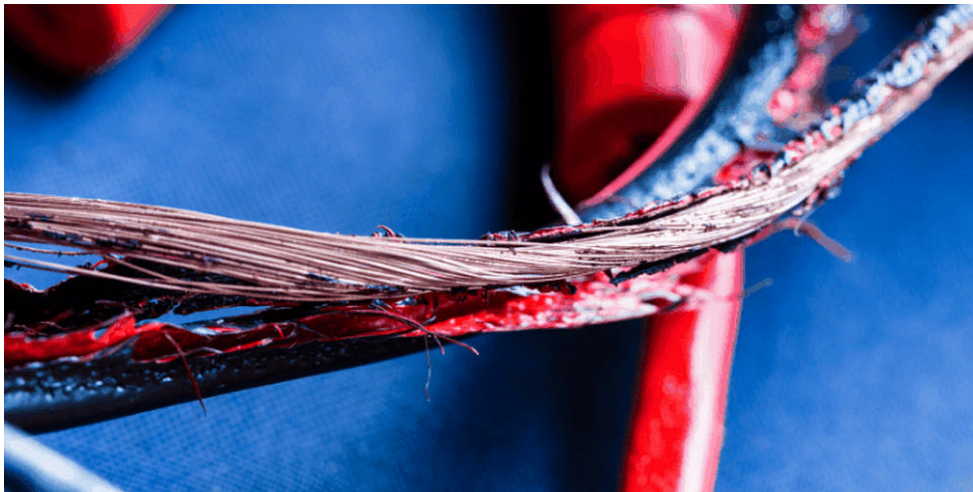
Figure 8: Overheating of electrical cables
