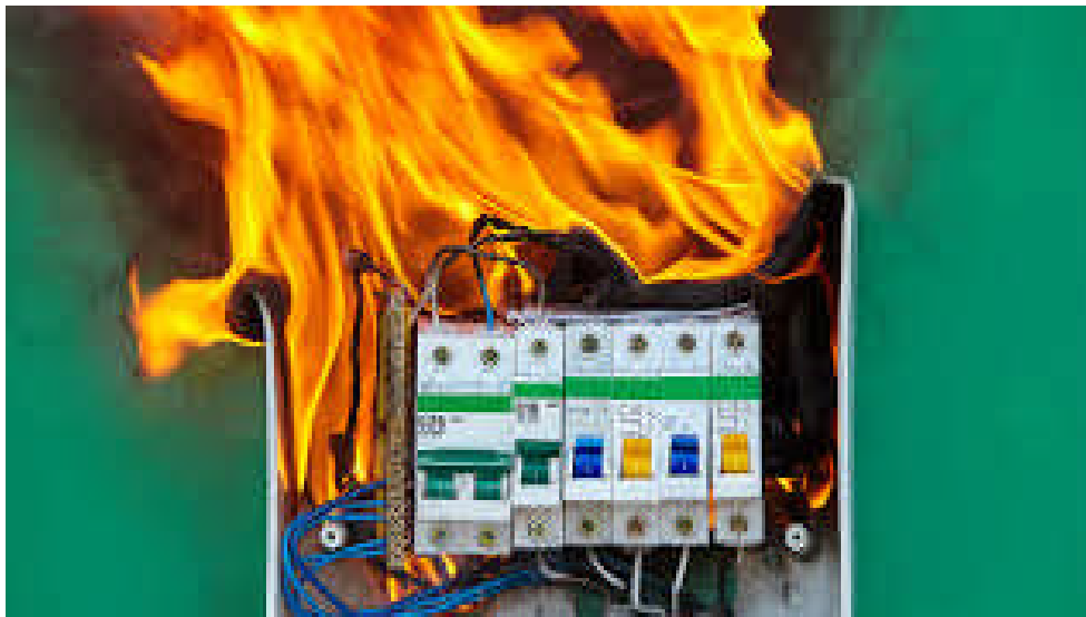
Figure 5: fire in an electrical panel
